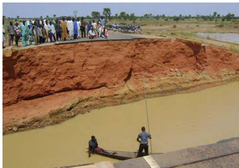
Post-disaster needs assessment, Nigeria, 2012.
