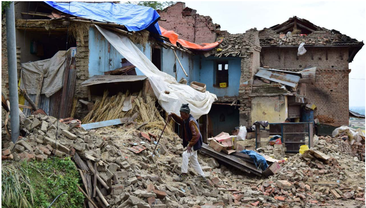
Damaged houses at Sudal village in Bhaktapur district, Nepal.
