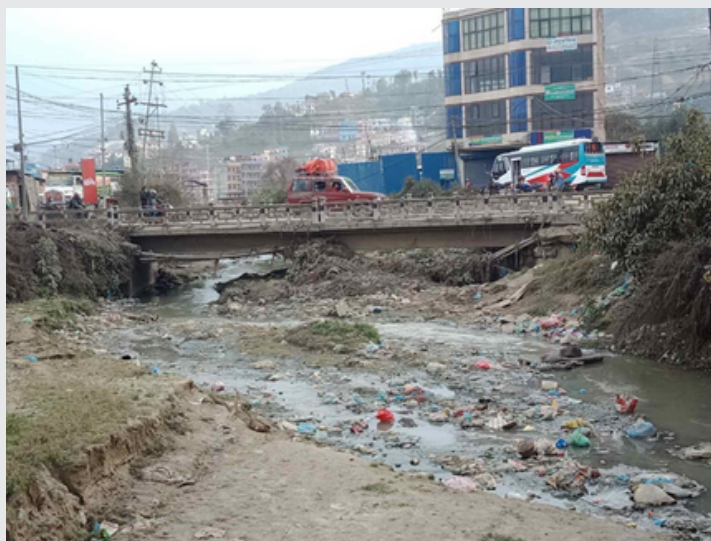
Depiction of low lying highway bridge in core area of the city Source: Nepal Red Cross Society
