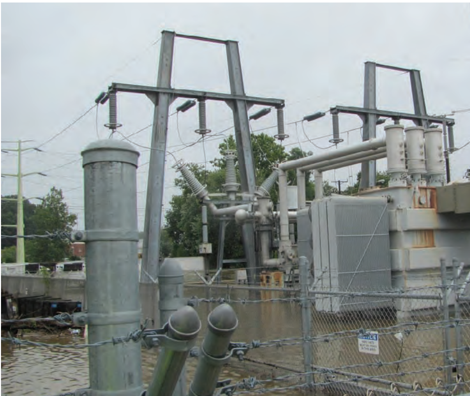
Figure E-04: Flooded substation (Flickr, FirstEnergy Corp, 2012)
