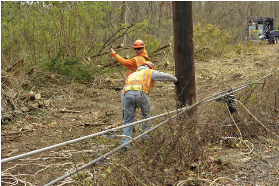
Figure E-06: A hard-to-reach distribution circuit that could be a candidate for selective undergrounding (NYPA, 2012)
