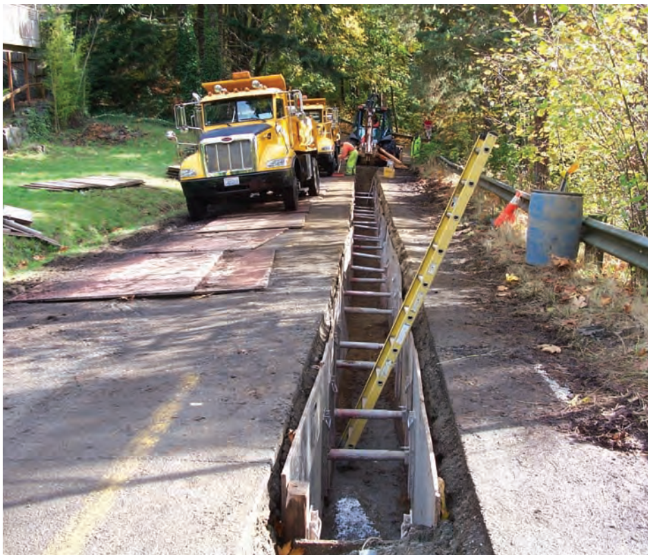
Figure E-07: A Seattle City Light project as an example of selective undergrounding of a power line with frequent outages (City of Seattle, 2012)
