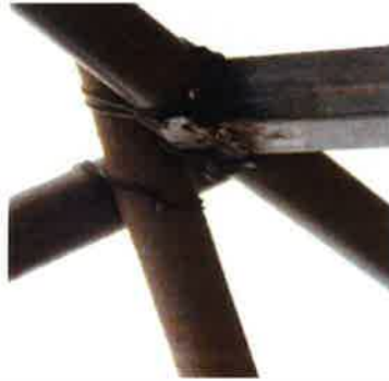
U-piece on the head of the vertical poles to ensure connection with the arch.
