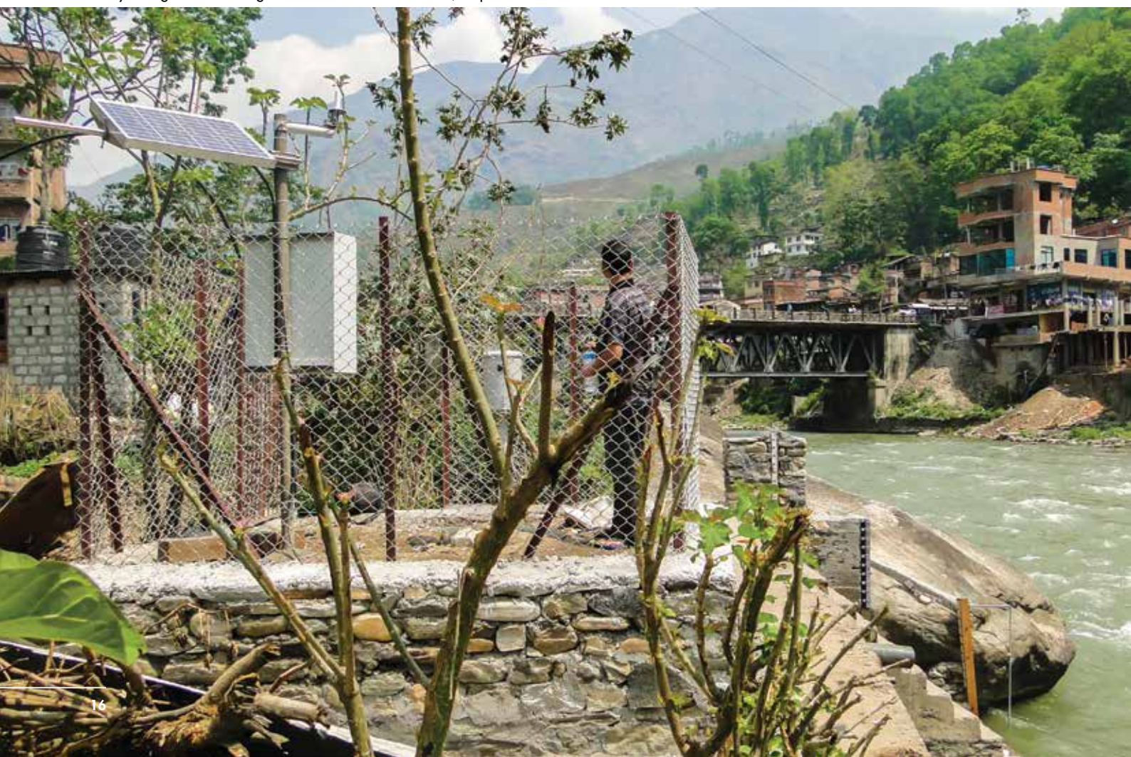
Hydrological monitoring station installed in Barabhise, Nepal
