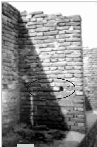
Figure 3.9: Weakness in building construction
