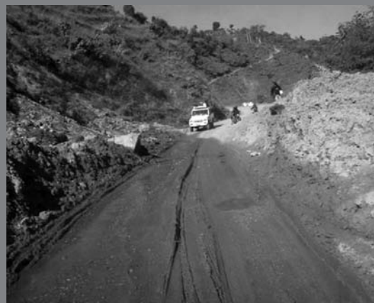
Landslide affected Dr. KI Singh Highway in Dadeldhura Photo Courtesy: Mohan Shahi, Kantipur National Daily
