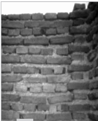
Figure 3.12: Improper bonding of masonry units
