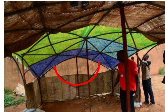
Bracing placed with a U shape in the short direction of the shelter
