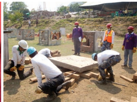
Fig.11: Lifting, moving and stabilizing heavy objects exercise during CSSRIW in Kurintar, Nepal, March 2014
