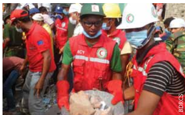
Bangladesh Red Crescent volunteers are cleaning debris at the collapsed Rana Plaza building.
