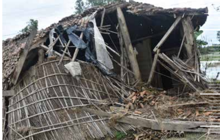
Damaged house in Samsi, Mahottari during July 2019 flood Credit: Bhesh Parajuli, Mercy Corps
