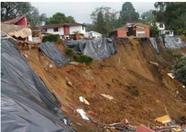
Figure 2: Slope Failure Source: Gonzalo Duque
