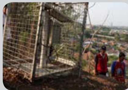
Landslide early warning system in Kelurahan Bendan Duwur village
