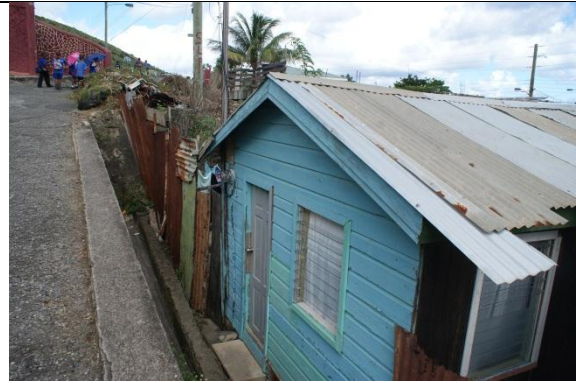
Road opposite catholic church where drainage runs off into houses in Dennery
