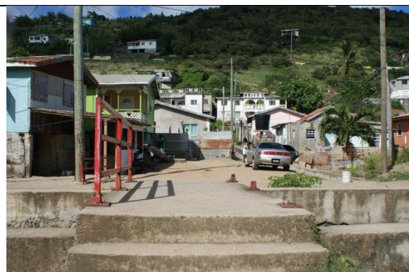
Damaged bridge in Dennery; one of the safety hand-rails was destroyed during floods.
