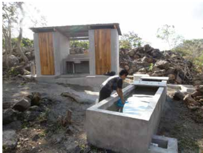
Photo: Bathing and washing facility, built with a water harvesting reservoir, Community of Malpaso
