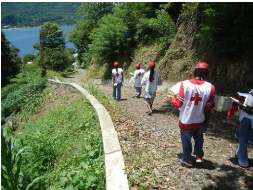
Example of a roadway (Lucy Vale Top hill) which turns into a flooded drainage course due to absence and poorly designed side drains to carry off surface water during rain downpours.
