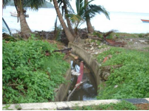
Above the drain is filled with garbage which outflow is to the sea coast. (Settlement village)
