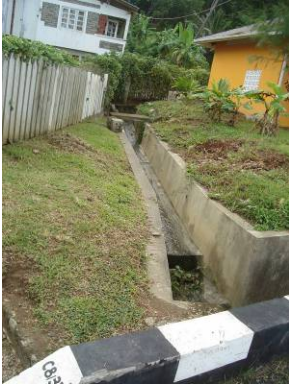
Storm drain along the Speyside Windward main Road that was reported that becomes flooded due to limited capacity during rain fall
