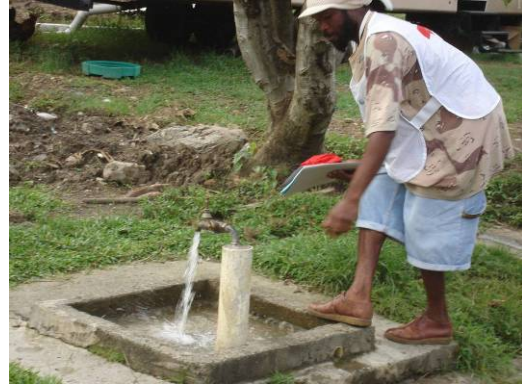
Example of a functioning public stand pipe
