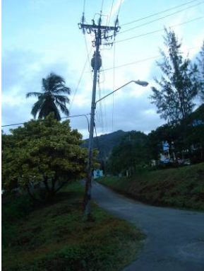
Examples of hazardous electrical poles
