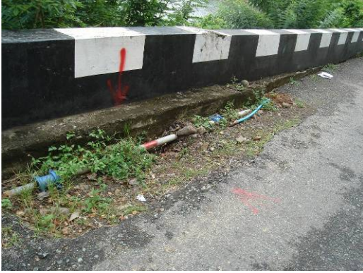
Exposed drainage pipe line along the road to Anse Bateau (Blue Waters Bay) which supplies Blue Waters Inn
