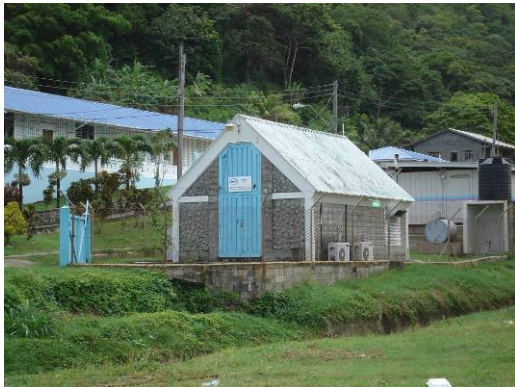
TSTT Phone communications hub system
