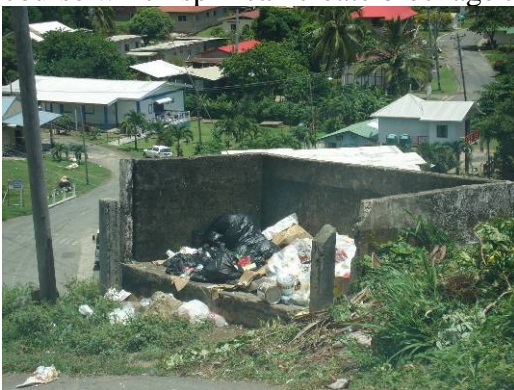
Examples of community sold waste collection facilities Lower Top Hill Note open garbage bin which is a health and safety hazard
