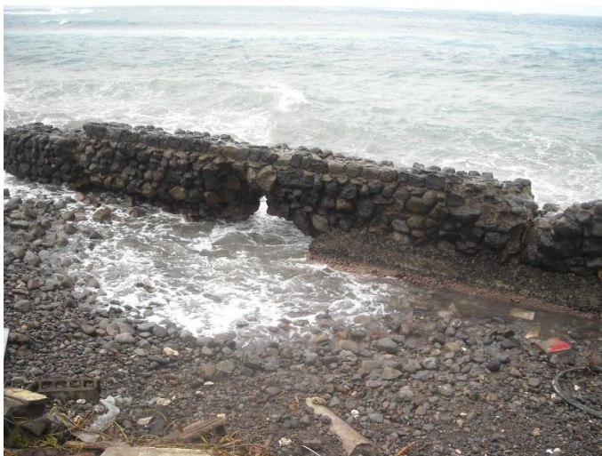
Figure 2 Coastal Erosion Dieppe Bay
