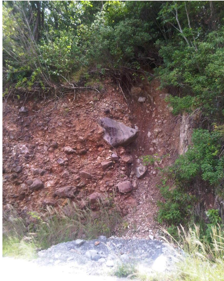
Location prone to falling trees and landslides
