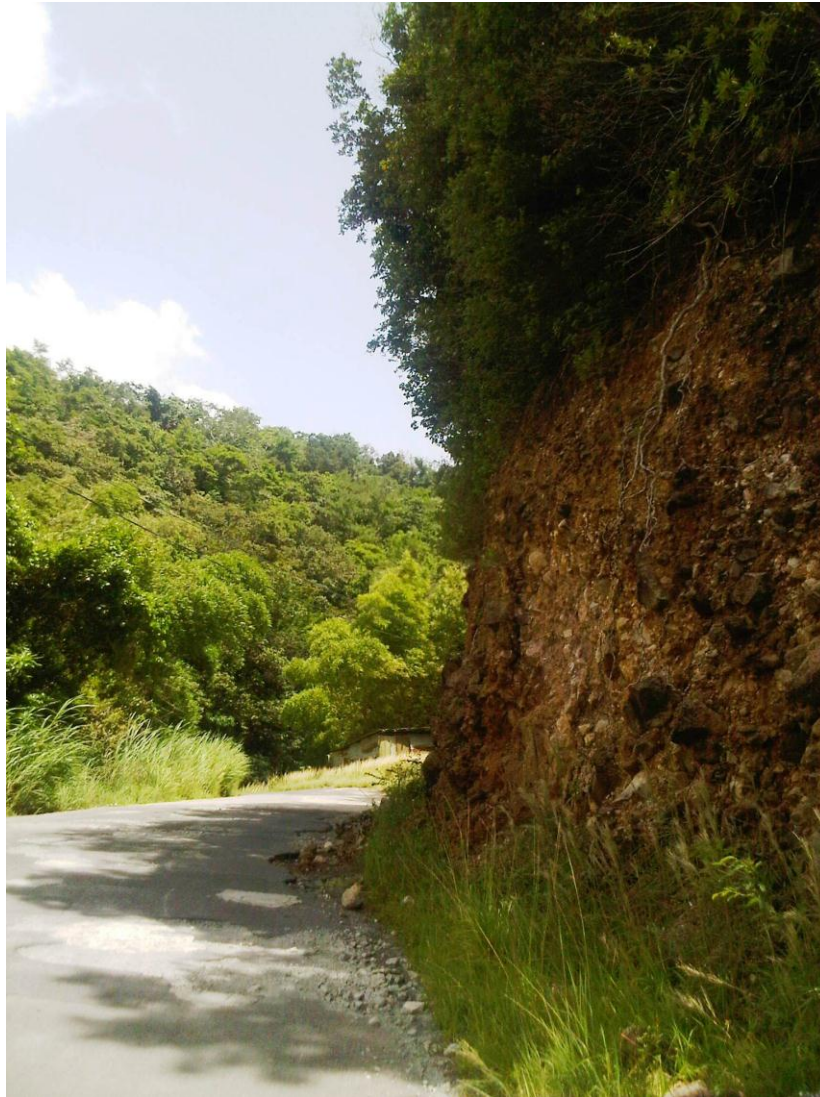
Rock Fall along Cochrane Road
