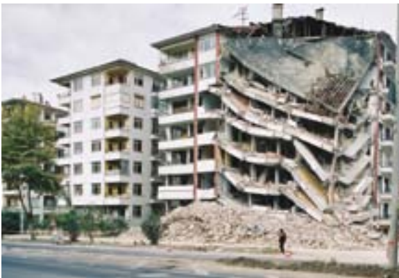
A multi-storey RC frame apartment house in Golcuk, Turkey partially collapsed by the 1999 earthquake. The lack of adequate moment connections and very thin columns is evident. © Randolph Langenbach
