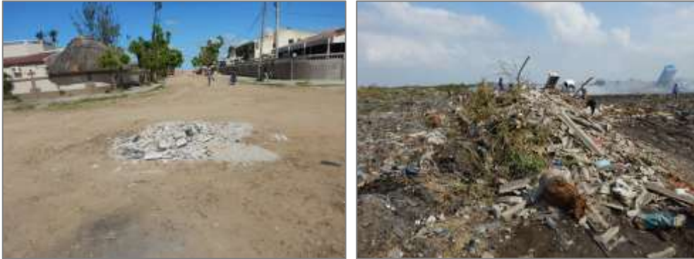
Figure 3 – Filling of potholes with asbestos cement rubbles and disposal at Beira dumpsite
