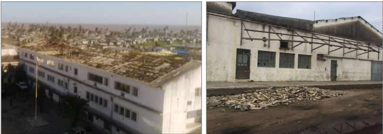
Figure 1 – Damaged fibre cement roofing in Publics and Commercial buildings in Beira city
