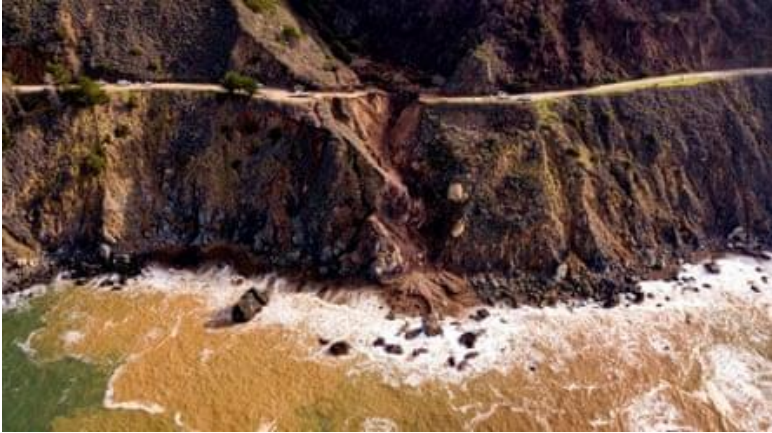
Image 1: Picture showing landslide causing a 150ft section of Highway 1 to wash away into the sea.
