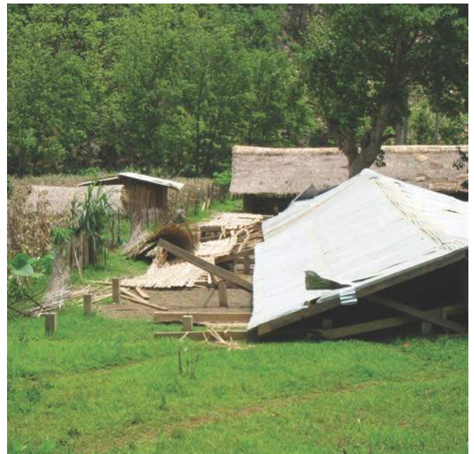
A community-built school in Laos, designed and constructed without sufficient technical support, collapsed in high winds. Several students were trapped but successfully rescued. Photo: Save the Children.
