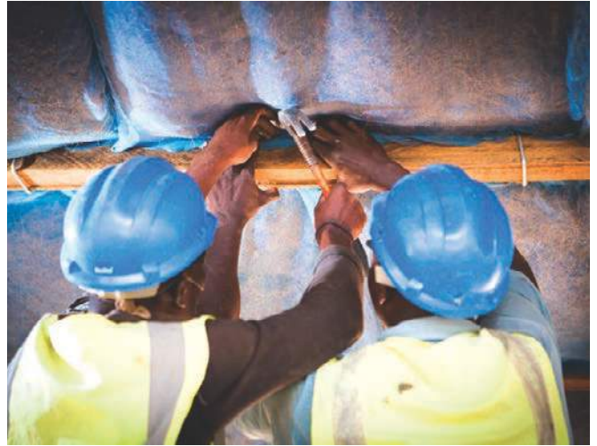
Local labourers install sacks of coconut husks in the roof for thermal and acoustic insulation. Photo: Jack Brockway.
