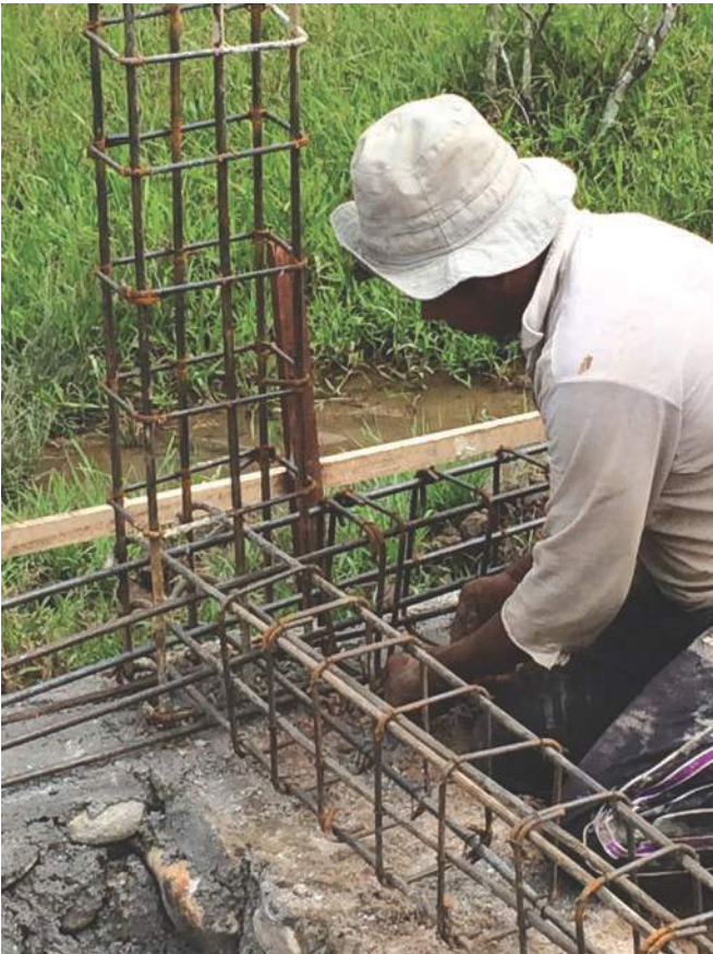
A local construction worker preparing the steel reinforcement prior to the pouring of concrete for a new school. Photo: Arup.
