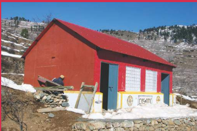
School reconstruction following a devastating earthquake in Pakistan deployed prefabricated steel panel elements that could be transported piece by piece and fixed to an in-situ reinforced concrete foundation. The prefabricated design enabled easier quality control of important structural elements and made best use of local resources. Photo: Joe Lapp/CRS.
