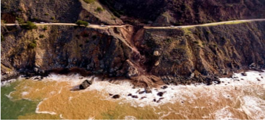
Figure 2: Landslide causing a 150ft section of Highway 1 to wash away into the sea. Source
