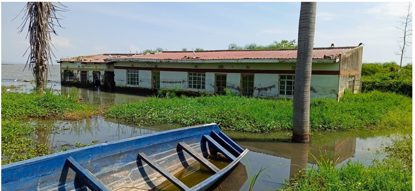
Image 6: A housing structure destroyed by floods
