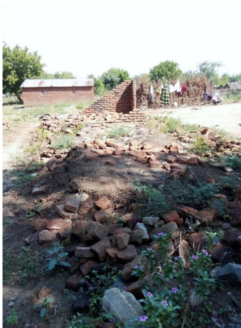
Figure 9: A house completely damaged by floodwaters following Cyclone Freddy. (Photo by the author)
