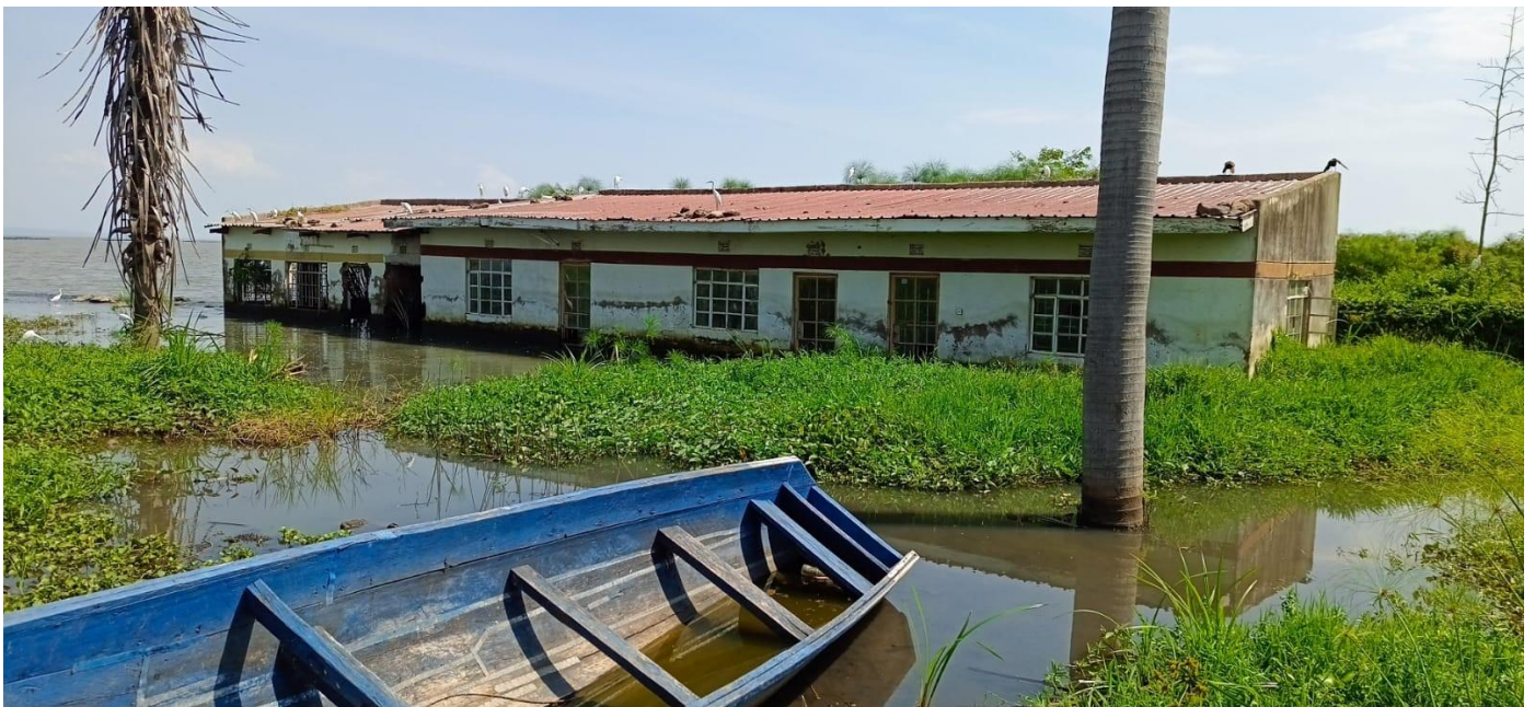
Image 6: A housing structure destroyed by floods
