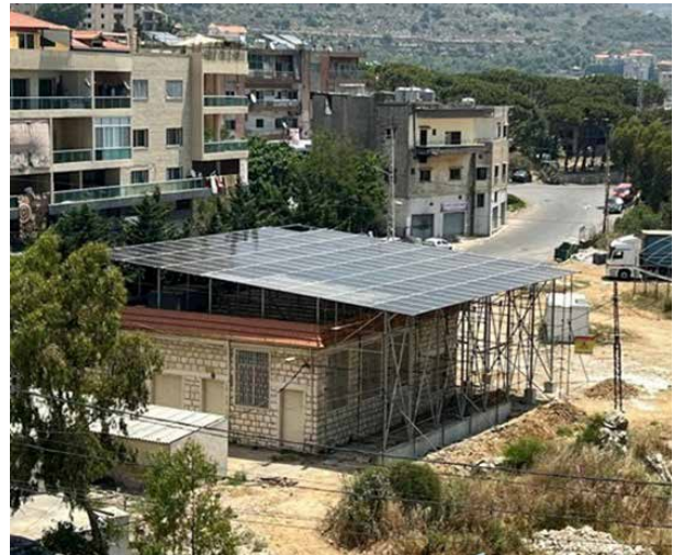
Solar systems installed by LRC to support host communities in Aley, Lebanon. Photo credit: Lebanese Red Cross.
